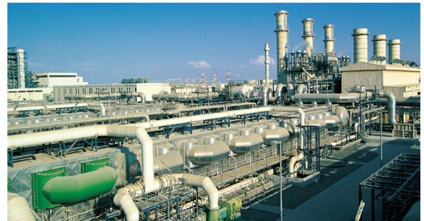
▲Desalination Equipment ( by Doosan Heavy Industries & Construction ) 海水淡水化装置(斗山重工業殿ご提供)
